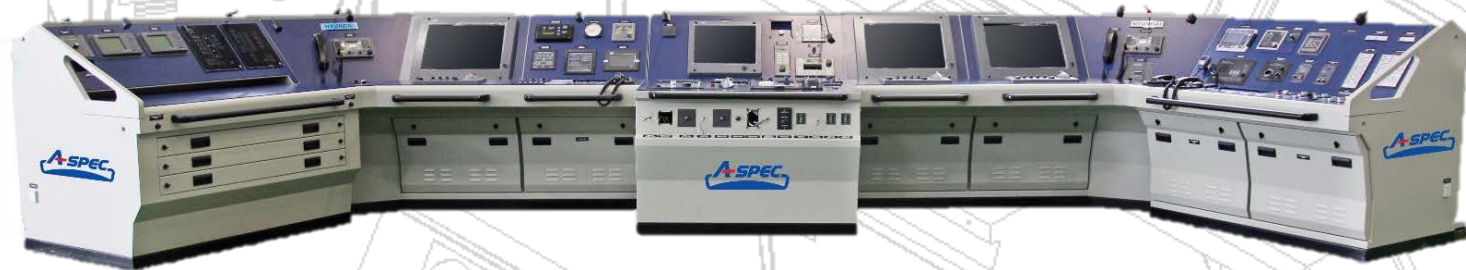
BRIDGE CONTROL CONSOLE
