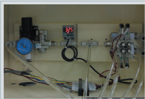
CLEAN CONVEYOR PNUMATIC COLTROL BOX
