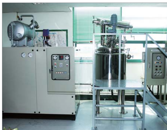
Polymerization Reactor System
