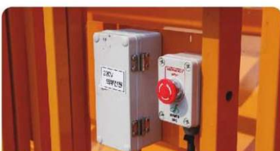
220V A/C POWER SOCKET PLATFORM
