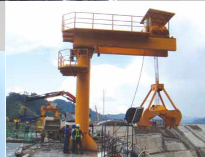
Jib Crane & Gorbelt Crane Bakun dam in Malaysia 10ton Arm 7m Jib Crane Max Capacity : 10 tons
