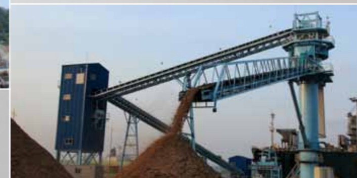
Cargo Unloading Plant Conveyor Crane (Woodchip) Harbor unloading System No. 7 South Entry in New Ulsan Port Capacity : 800 tons / Hr
