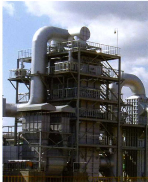
LCD Incinerator Wet ESP.
