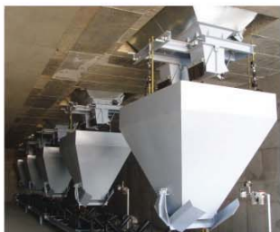
터널 저장빈 & 계량빈 Tunnel Storage Bin & Weighing Bin
