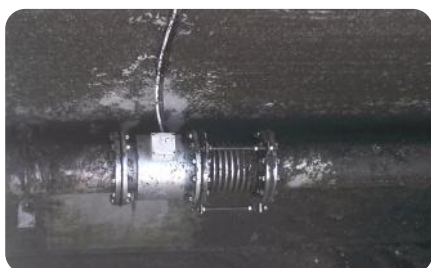
Seosan Disposal Plant of Sewage
