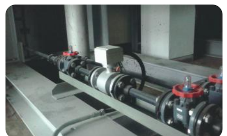
Suncheon Disposal Plant of Sewage
