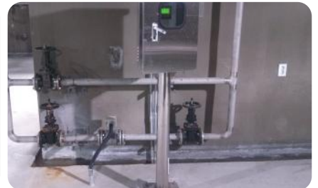
Tancheon Disposal Plant of Sewage
