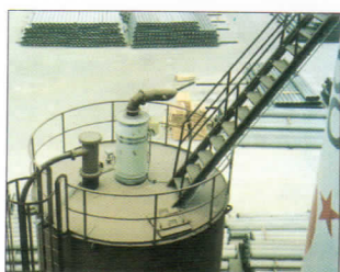
• BAG FILTER & FEEDING PIPE
