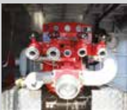
Water Pump / Foam system
