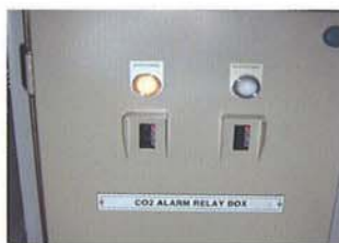
▲ Alarm Relay Box
