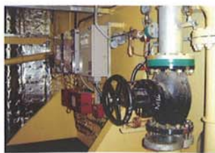
▲ P.O.D Valve Assembly (Main Isolating Valve)
