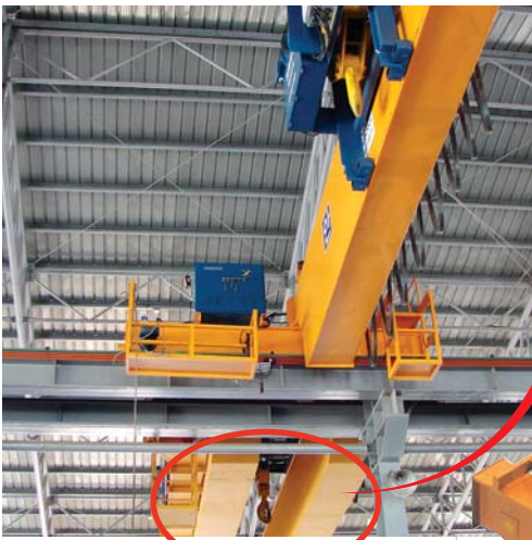
■ DHO 20 tons Span 20m
