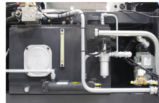
Independent filtering & cooling system
